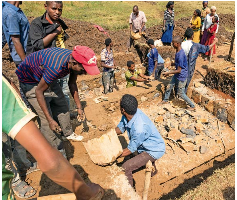
Participation from the outset: In all our projects, as here in the construction of a spring development, we actively involve the local population.
