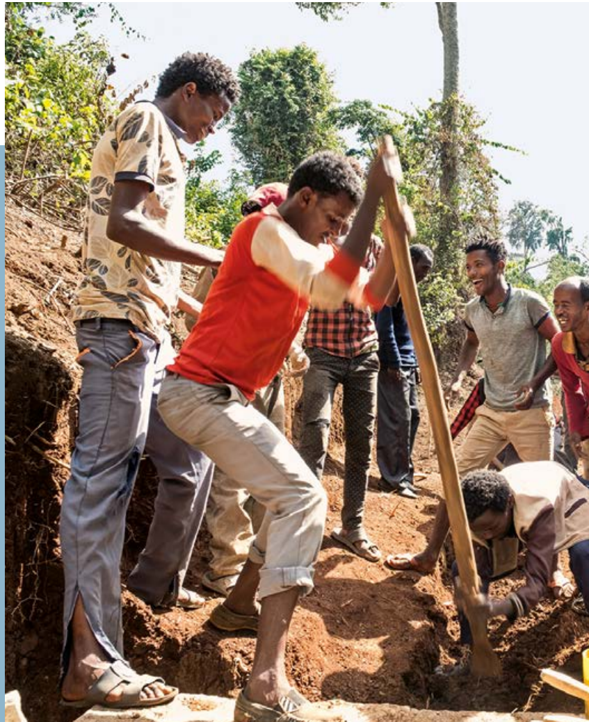
With many helpers, the ditches for the water pipes are soon dug.
