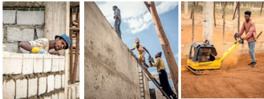
The construction site for the TVET in Bure is progressing in leaps and bounds.
