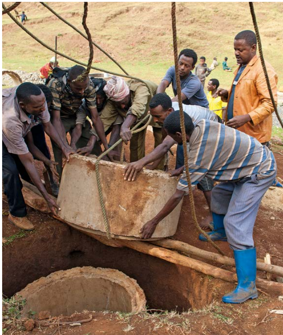
Borecha project region: there is no lack of help for installing the last well ring.
