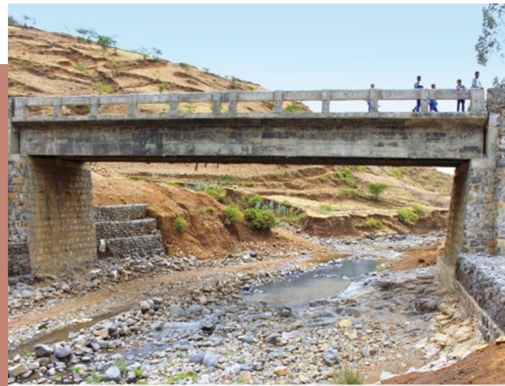
In the rainy season the Kulbit River becomes a raging torrent, but the new bridge provides a safe crossing.
